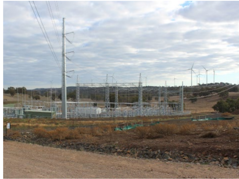
Image 2 Typical Substation (Source: NGH)
