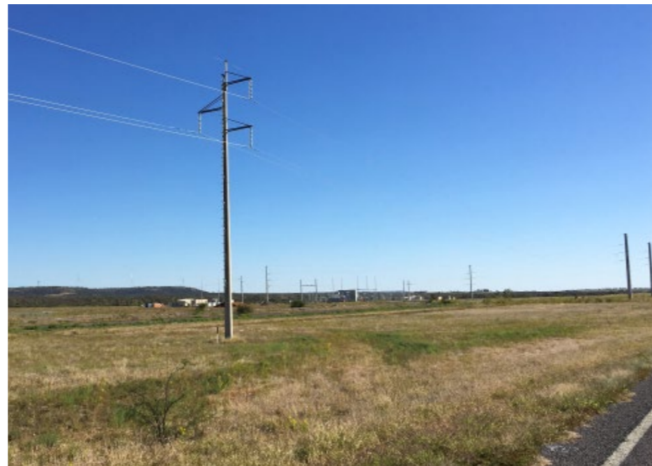
Image 4 Transmission Line (Source: NGH)
