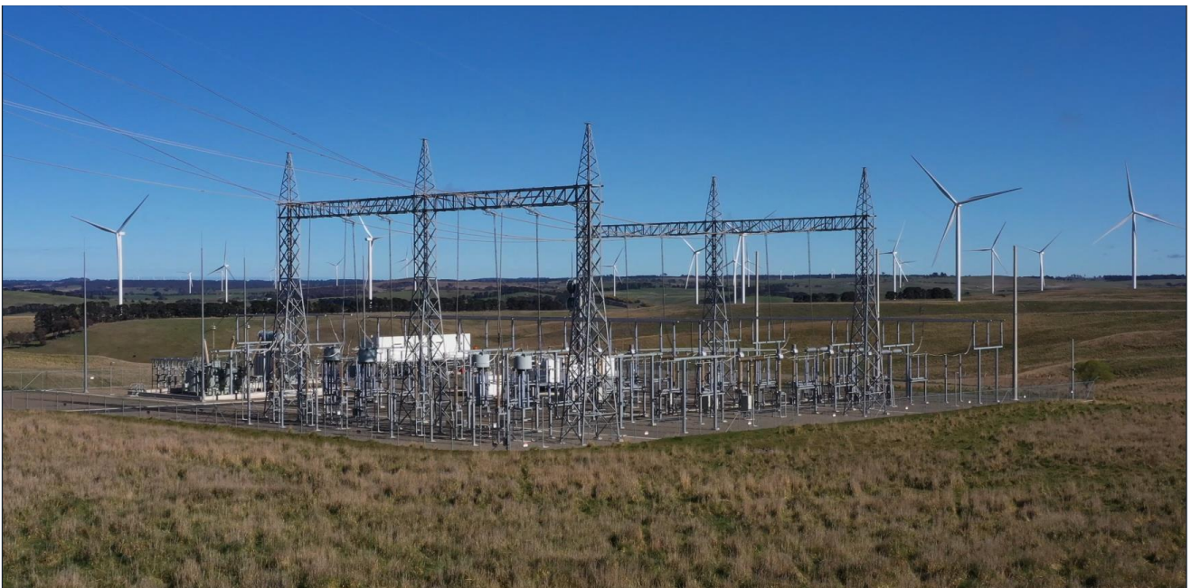
Figure 20. Image showing transformer, circuit breakers, gateways and surge arresters (Source: GPGA, 2022)
